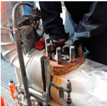
Trim installation into existing valve at customer site
